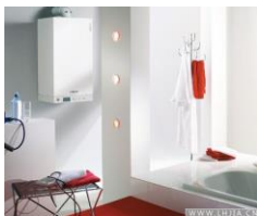
Wall Mounted Natural Gas Heater
