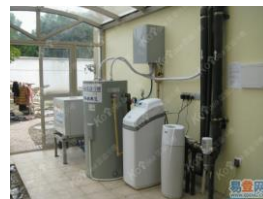
Geothermal heat pump
