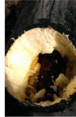
Fig. 2 - Moisture spread, stemming from a casing joint, damaged by large movements.
