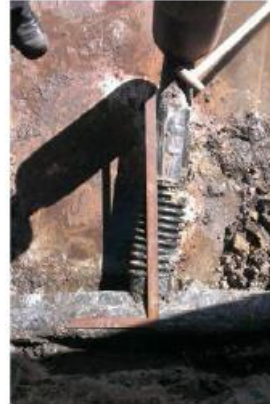
Fig. 1 - Branch, damaged by large movements.
