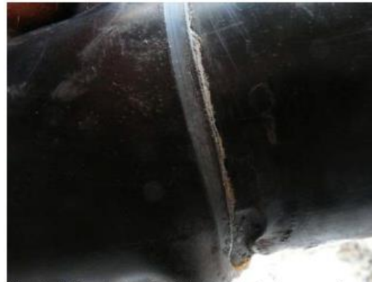
Fig. 5 - Dislocated casing joint due to the large number of movements
