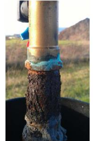
Fig. 3 - Released copper ions from brass valve, causing corrosion of the steel pipe. The damage is on the return pipe. No damage on the flow pipe.
