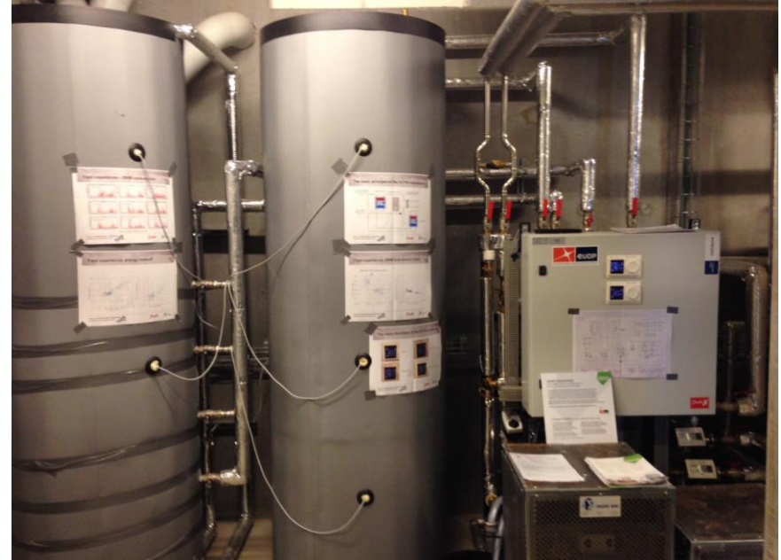
Installed at Nordhavn site
