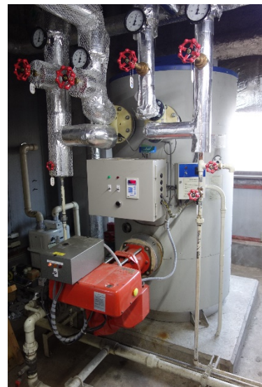
LP Gas Boiler(460kW)
